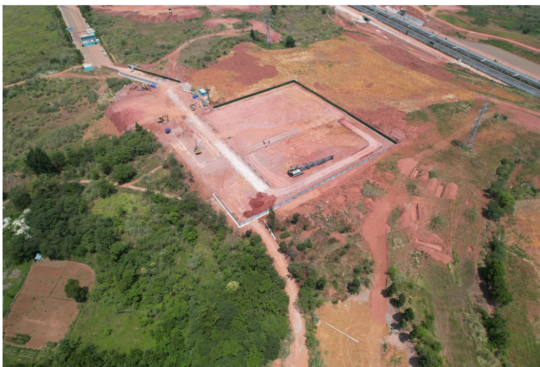
图3-3变电站区无人机航拍
